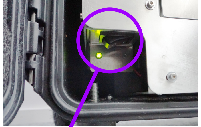
Main switch inside the case
