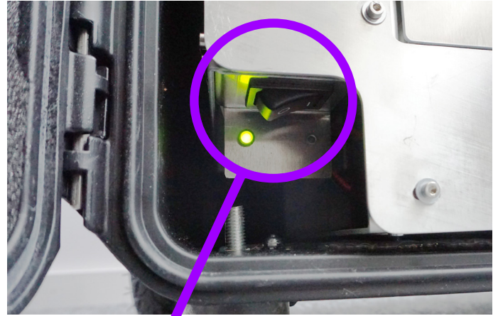
Main switch inside the case
