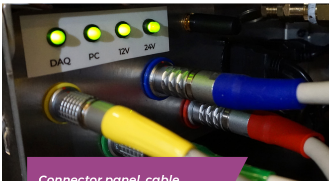
Connector panel, cable connections and indicator leds inside the case
